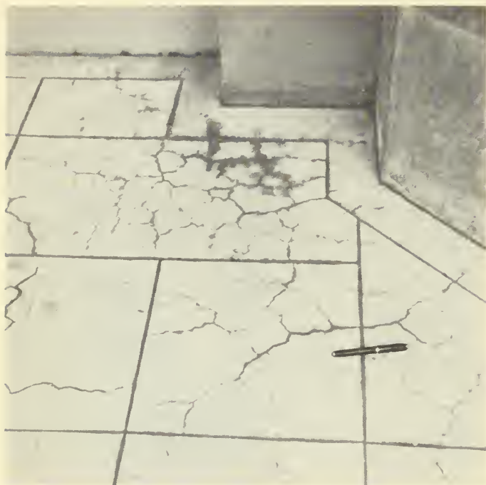
FIGURE 9. Pattern cracking in floor, Law Building, University of Southern California, Los Angeles.
